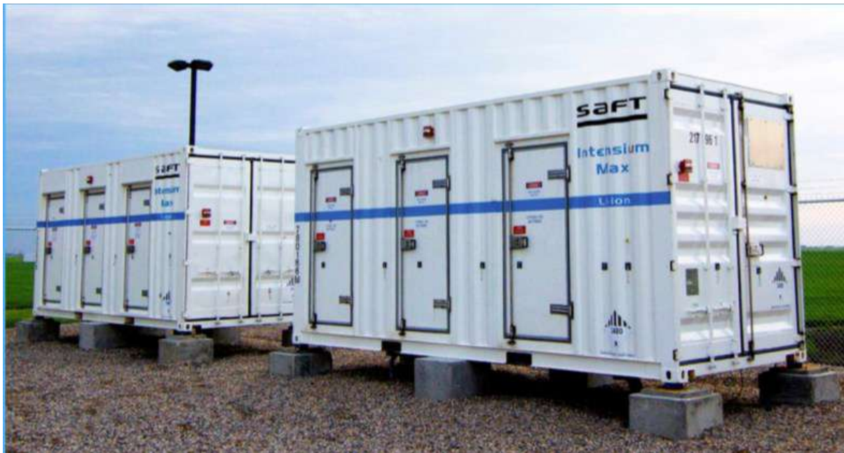
Figure 6-2 Typical battery containers used on a solar farm
